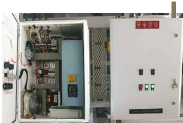
Windlass control panels with frequency converters
